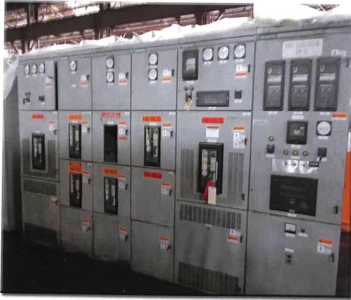
(2) RL4200, (4) RL1600 AIR CIRCUIT BREAKERS
