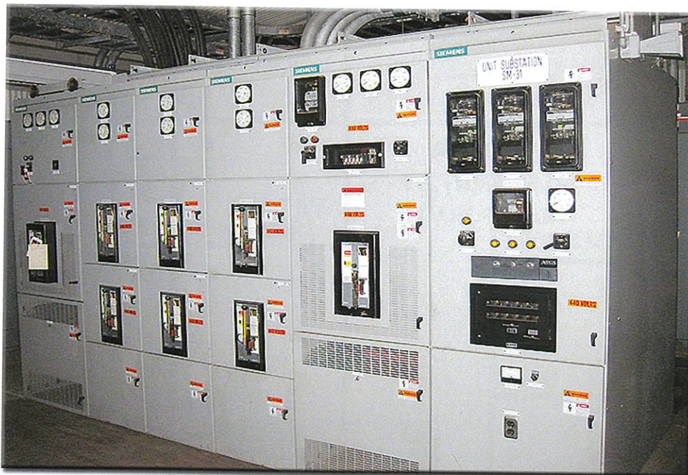
(2) RL4200, (3) RL2000 AIR CIRCUIT BREAKERS
