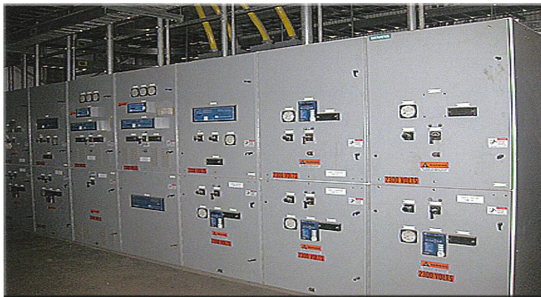
5 KV SIEMENS 5 GMI (3) 2000 AMP 5-GMI-350-2000-78 (8) 1200 AMP 5-GMI-350-1200-78 VACUUM BREAKERS
