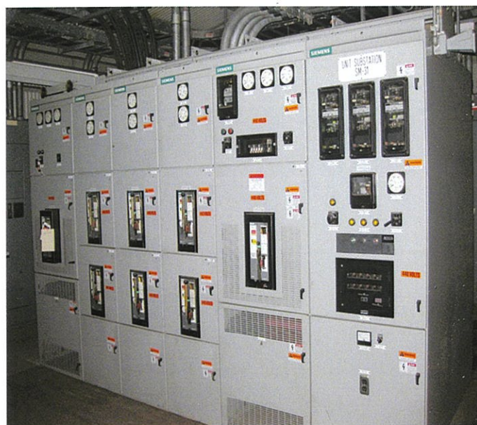
(2) RL4200 (2) RL3200 (4) RL1600 AIR CIRCUIT BREAKERS
